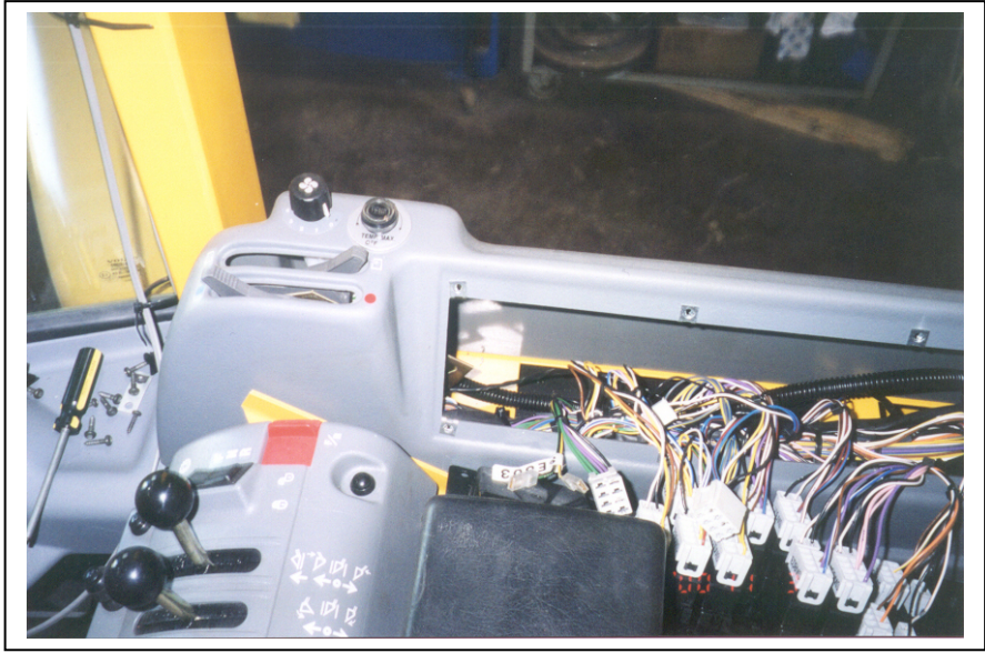
Thermostat mounted on L70D
